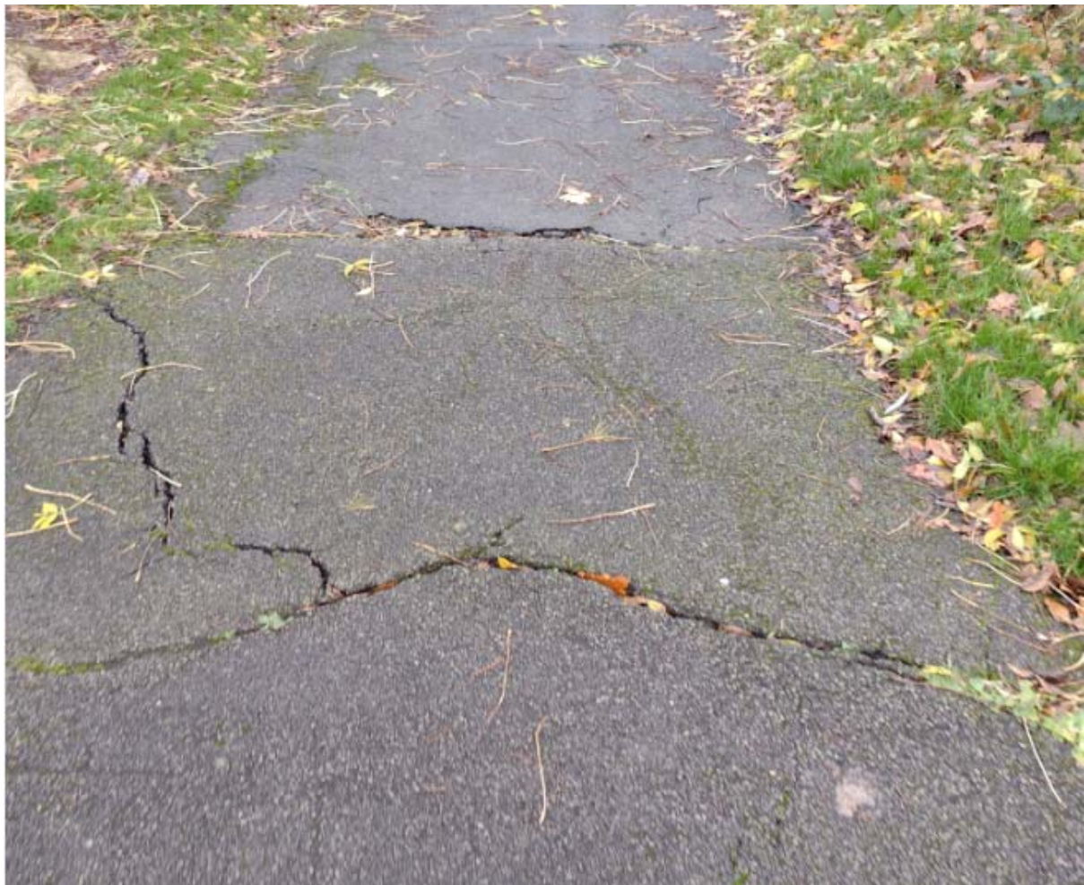
Europa Avenue Middleway footpath is in poor condition and a potential trip hazard
